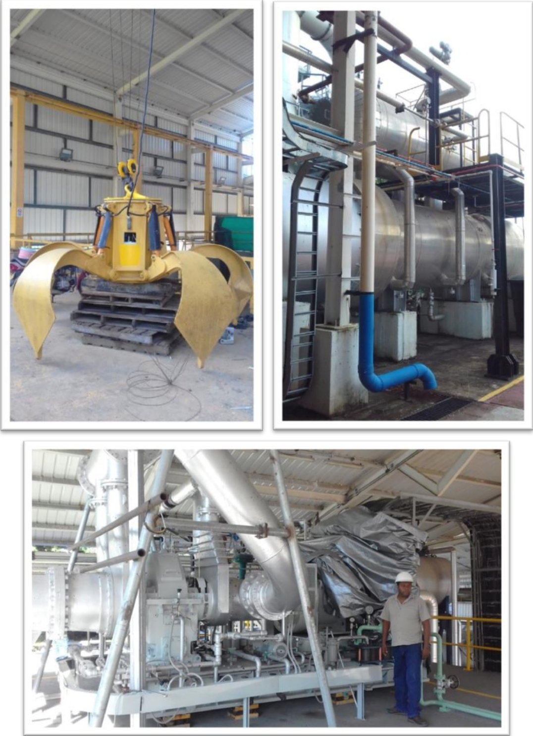
Some aspects of the WTE plant in San Andres
