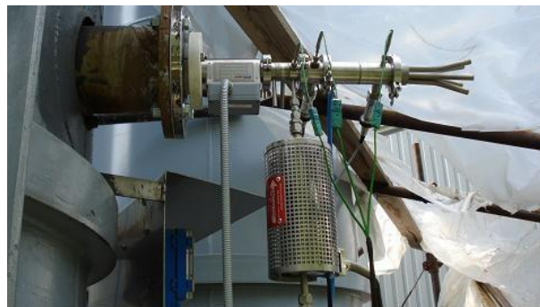
UF particulate sampling system in conveyed streams
